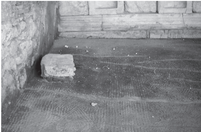
FIGURE 4 Sagalassos, Neon Library. Grouting of the cracks with cement mortar, general view (1996). Photo by Y. Selçuk Sener.
