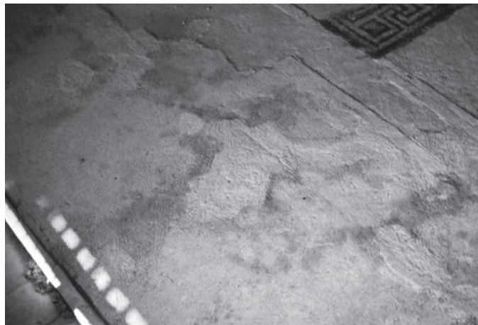
FIGURE 2 Aizanoi, Roman bath. Localized wet surfaces due to active rising damage (1994). Photo by Y. Selçuk Sener.
