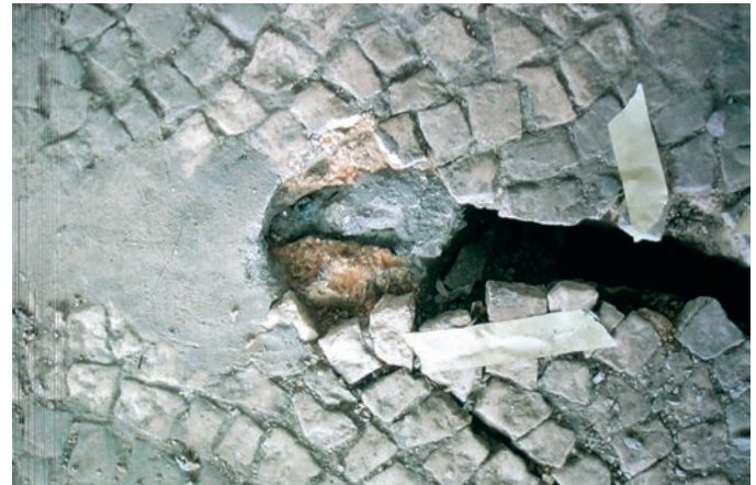
FIGURE 5 Sagalassos, Neon Library. Grouting of the cracks with cement mortar, detailed view (1996). Photo by Y. Selçuk Sener.
