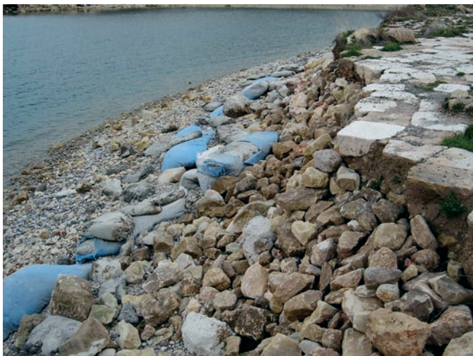
FIGURE 6 Zeugma. Condition of the shoreline where the mosaics have been reburied (2004). Photo by Y. Selçuk Sener.
