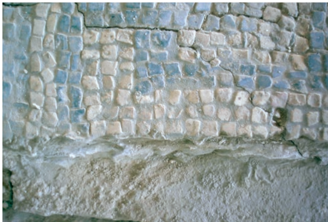
FIGURE 1 Aizanoi, Roman bath. Filling of interstices with cement mortar (1994). Photo by Y. Selçuk Sener.
