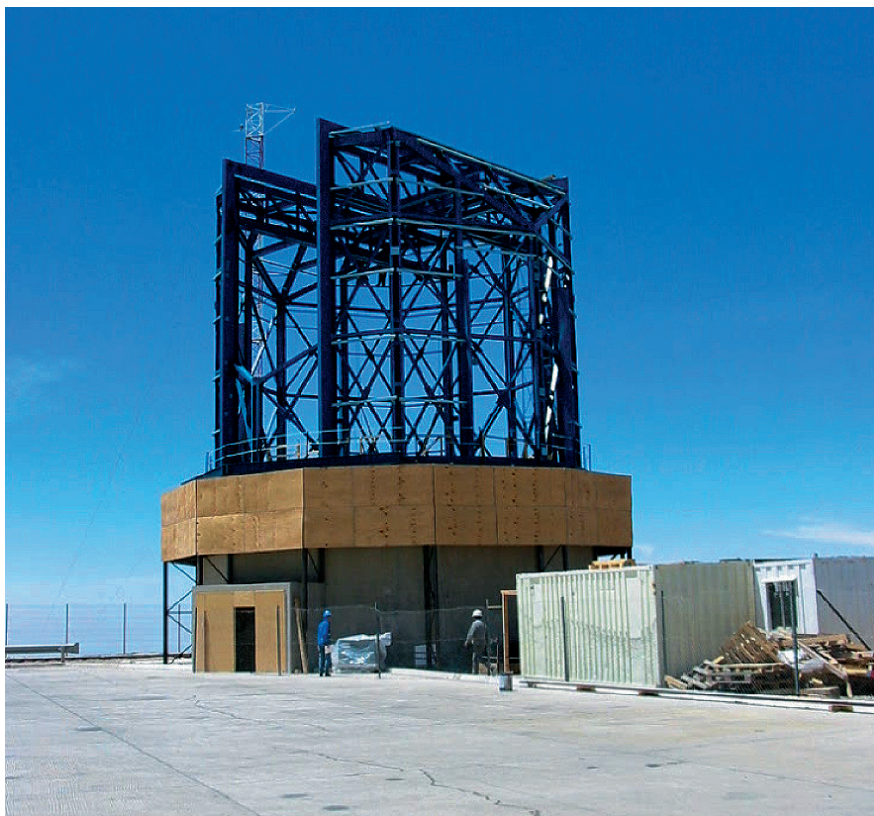
Figure 1: The VST enclosure taking shape at the edge of the Paranal platform.
